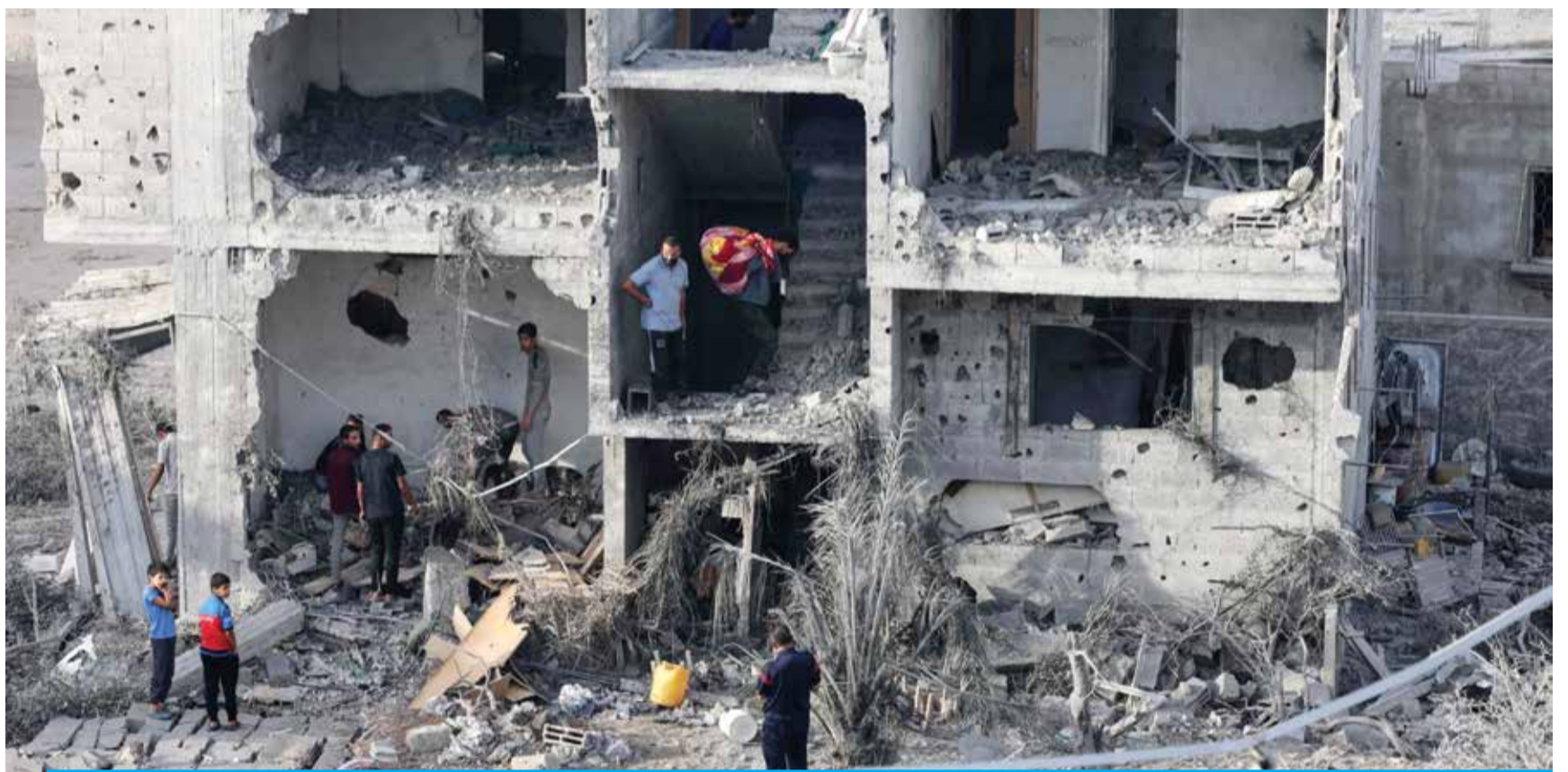
GAZA: People salvage some belongings from a damaged building following Zionist bombing on Rafah in the southern Gaza Strip on Nov 11, 2023. — AFP
