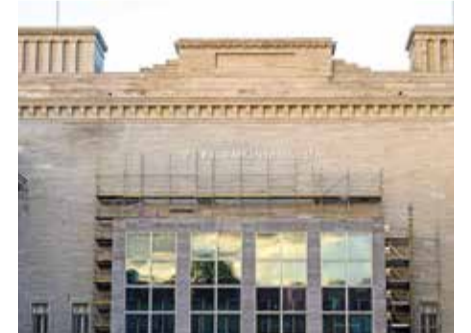
A general view shows the main entrance to The Pergamon Museum in Berlin as renovation works on progress.
