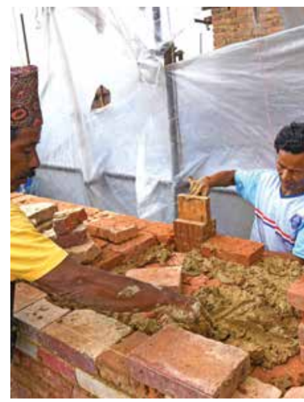
In this photograph laborers work at a reconstruction site in the Patan Durbar Square of Lalitpur district on the outskirts of Kathmandu.
