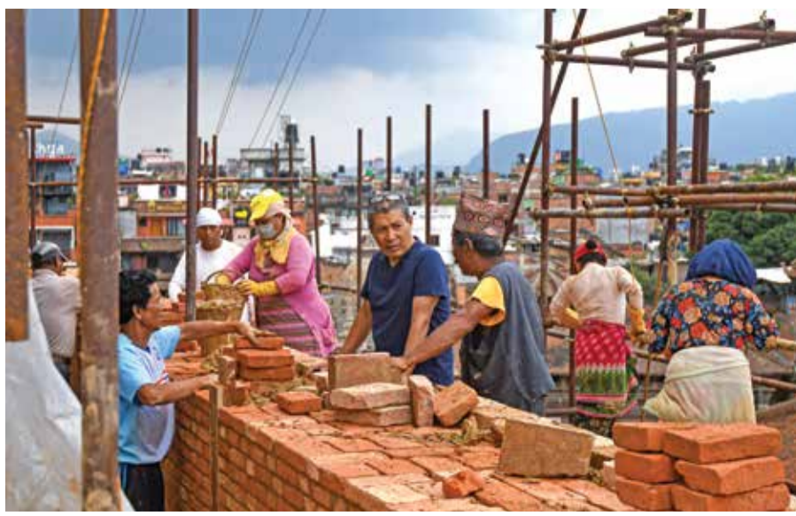
In this photograph heritage conservationist and Kathmandu Valley Preservation Trust director Rohit Ranjitkar (fourth right) speaks with laborers at a reconstruction site in the Patan Durbar Square of Lalitpur district on the outskirts of Kathmandu.
