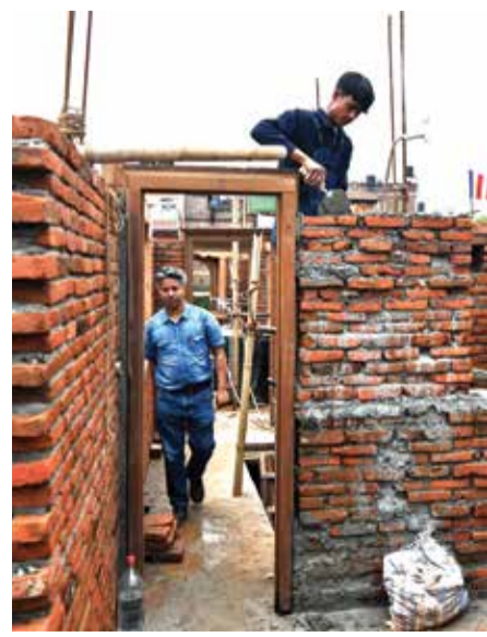
In this photograph heritage conservationist and Nepal Vocational Academy founder Rabinendra Puri (left) walks past a laborer working to reconstruct a temple in Bhaktapur.
