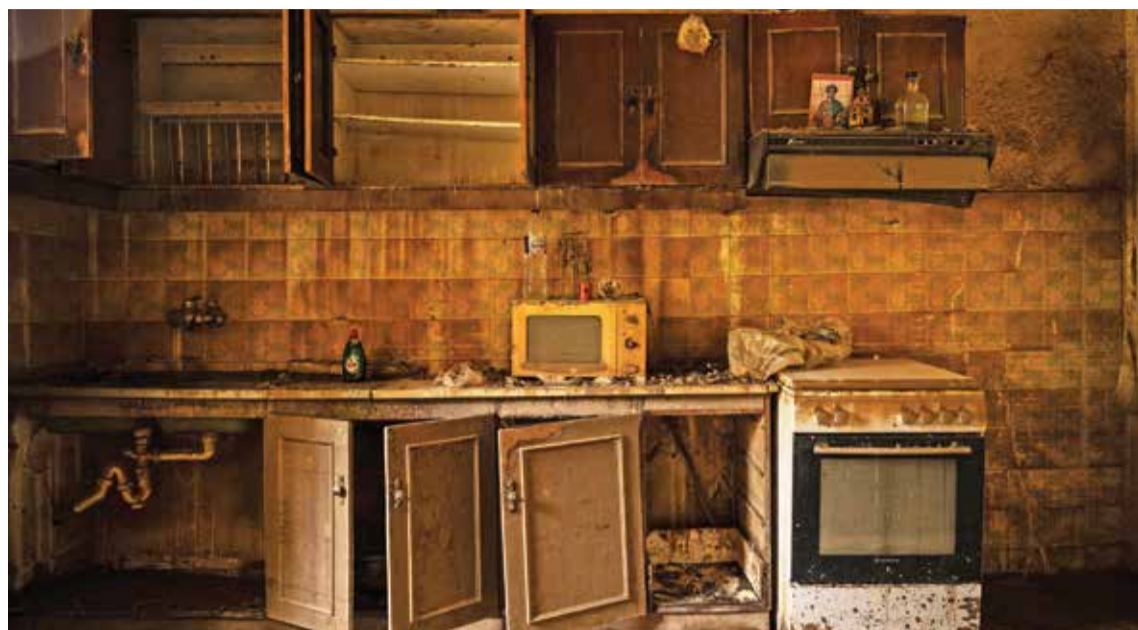
VLOCHOS: This photograph taken on Sept 25, 2023 shows the kitchen of a devastated house after the floodwater from Storm Daniel receded, in the village of Vlochos, central Greece. - AFP photos
