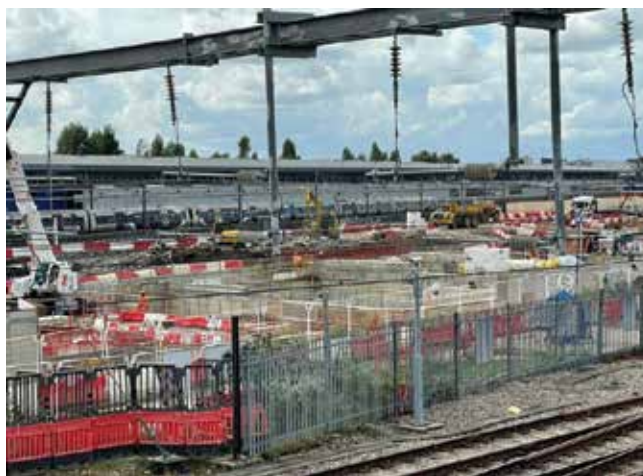
Work on the first section of HS2 began in April 2020, with the first trains due to run between 2029 and 2033.
