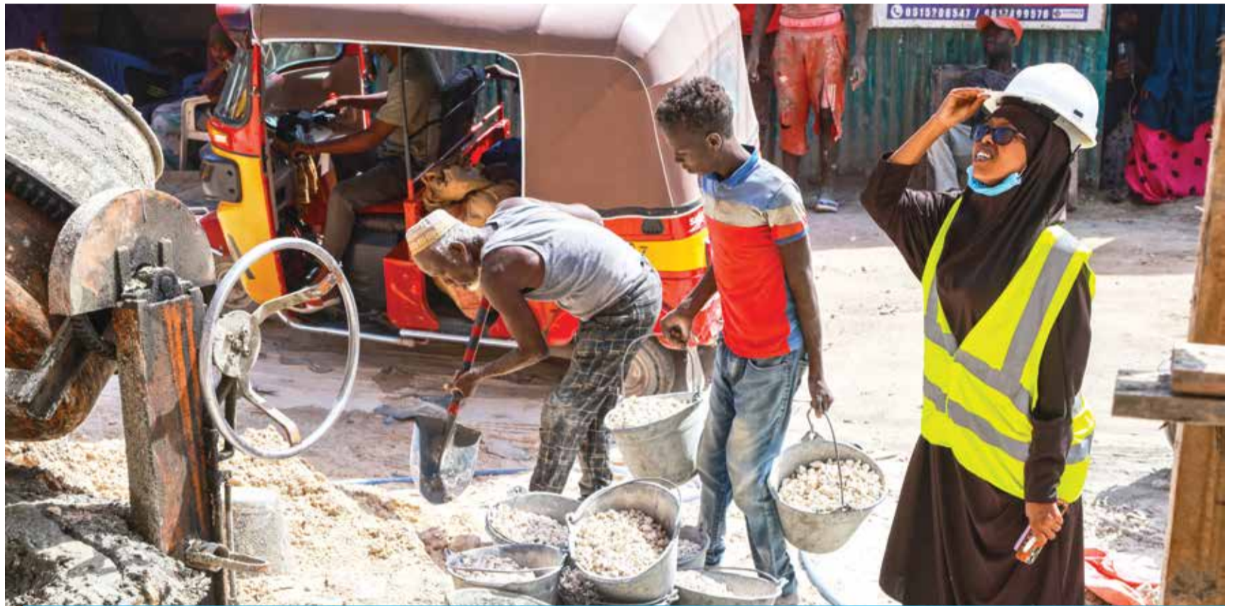
MOGADISHU: Civil engineer Fathi Mohamed Abdi (right) holds her protective helmet as she supervises a construction site in Mogadishu, Somalia on August 13, 2023.-- AFP
