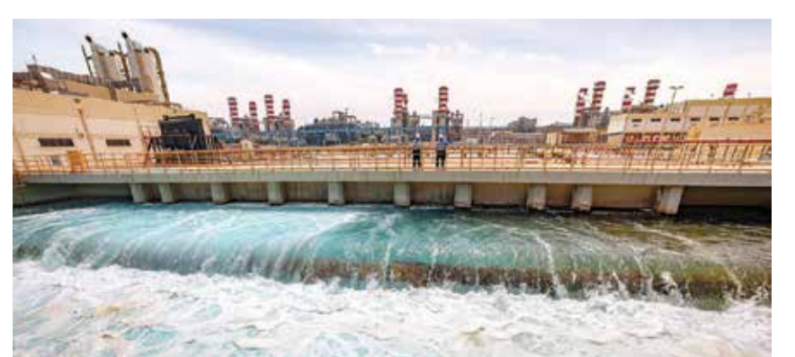
RAS AL-KHAIR, Saudi Arabia: Picture taken on March 30, 2023 shows the Ras al-Khair water desalination plant along the Gulf coast. — AFP
