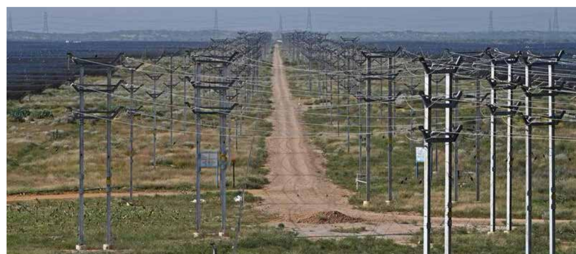
Solar electric lines at a park in Rajasthan. Saudi Arabia and India signed more than 50 agreements in September covering sectors including energy. — AFP
