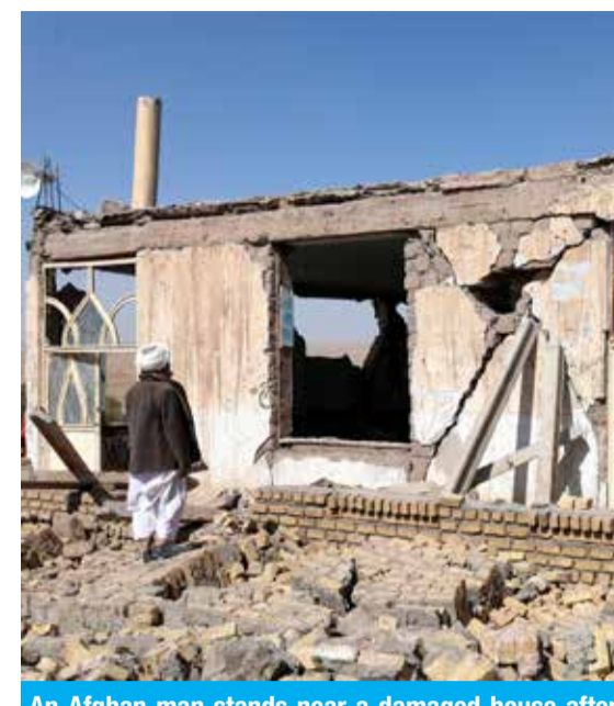
An Afghan man stands near a damaged house after the earthquakes in Sarbuland village.
