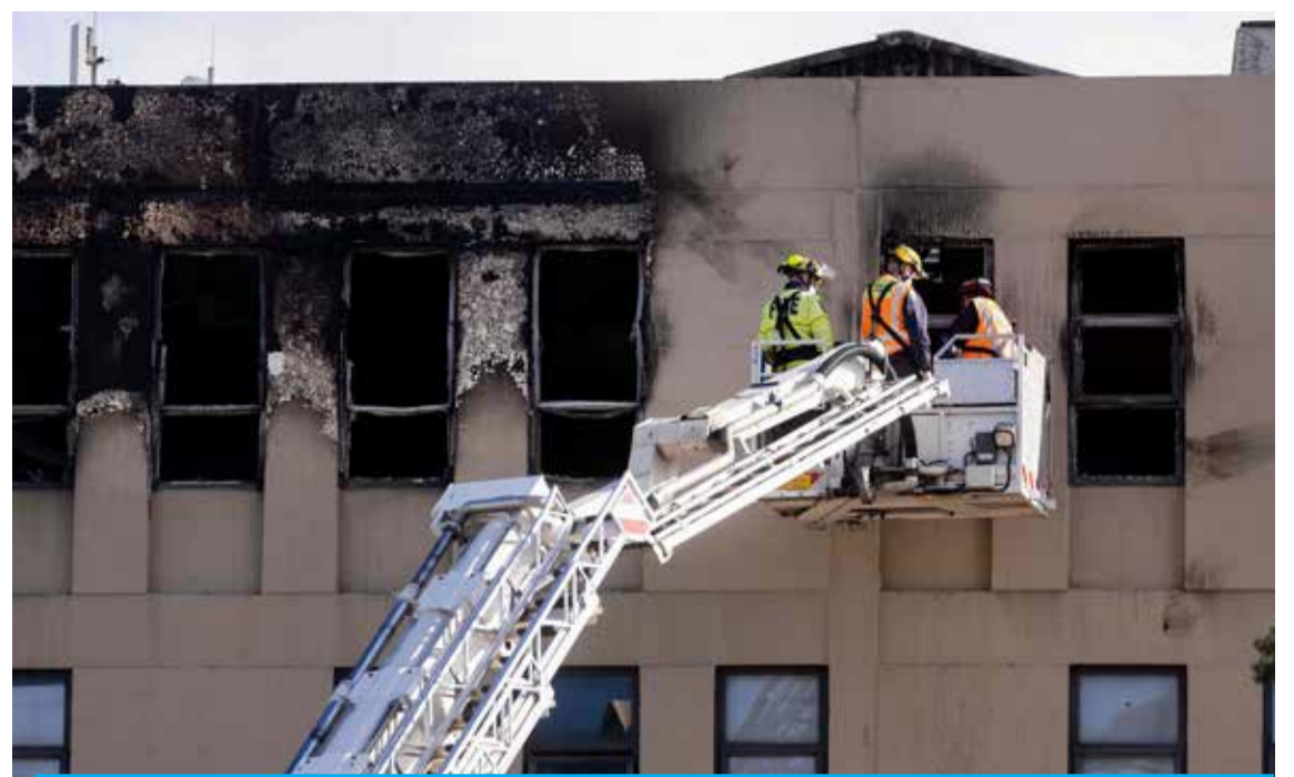
WELLINGTON: Firefighters inspect the Loafers Lodge hostel where a fire broke out a day earlier in the suburb of Newtown in Wellington. — AFP
