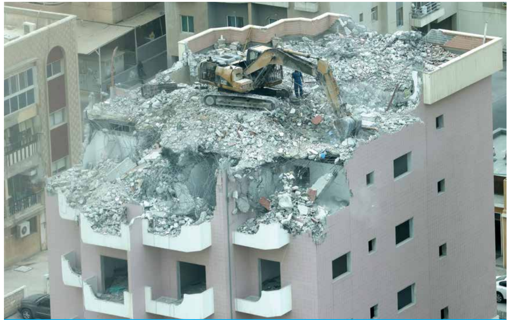
KUWAIT: A rooftop excavator tears down a residential building. — Photo by Yasser Al-Zayyat
