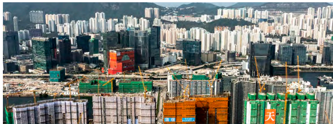
HONG KONG: This picture taken in Hong Kong on April 28, 2023 shows multiple under construction buildings (bottom) wrapped in bamboo scaffolding. The world's most skyscraper-laden metropolis is also one of the last remaining major cities to use bamboo scaffolding for modern construction and building repair. — AFP
