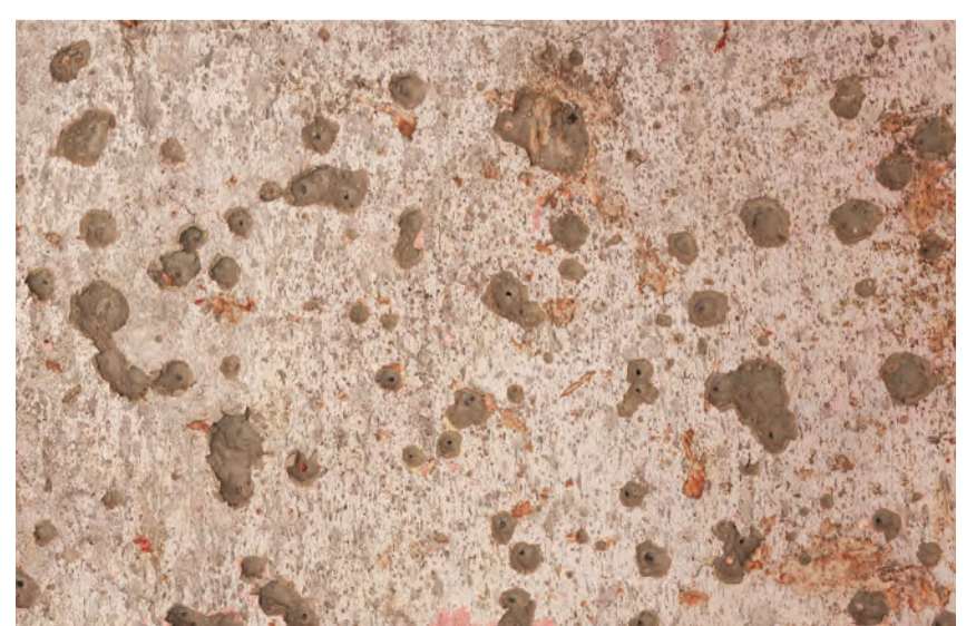
NABLUS: Bullet holes riddle a wall at the site where three Palestinians were killed, during a raid in the occupied West Bank city of Nablus on May 4, 2023. — AFP
