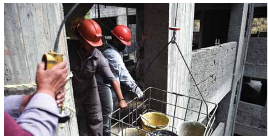
Women workers unload buckets of cement by a rope-driven mechanical device to lift heavy loads during the construction of the residential building "Jorge Rodriguez Padre" in the Algodonal community in Caracas.
