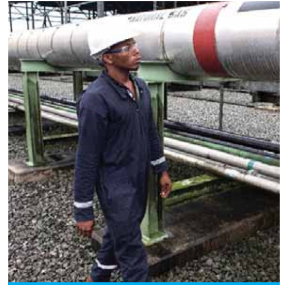
A gas pipeline at a power plant in Nigeria.
