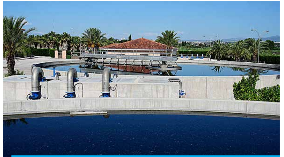
LAS TORRES DE COTILLAS: Photo shows a view of a sewage recycling plant of EDAR company, recycling water for agriculture, in Torres de Cotillas near Murcia, southern Spain. — AFP
