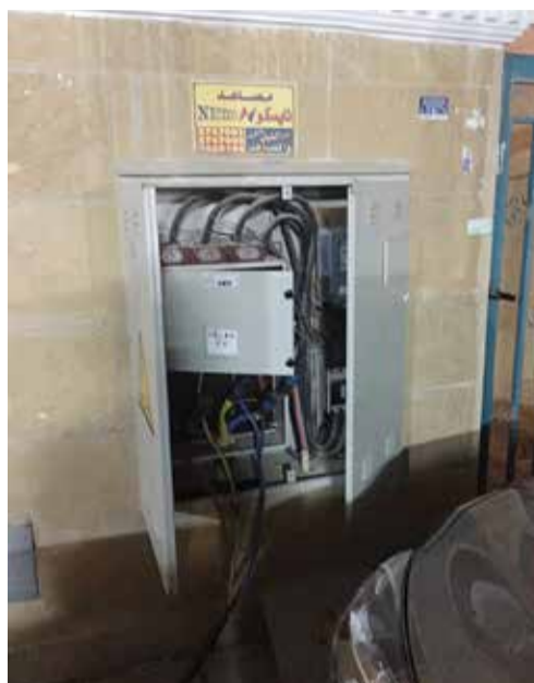
A power box placed at the front of one of the buildings on the street was left wide open for hours after workers connected it to one of the generators.
