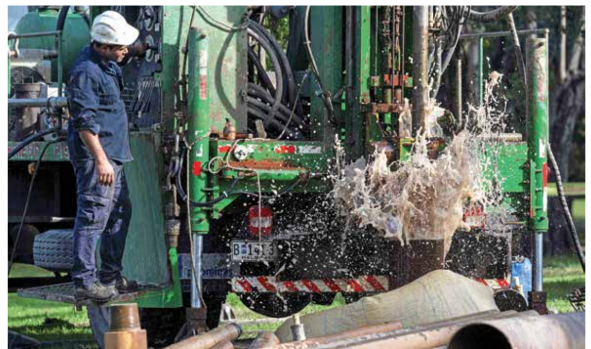
MONTEVIDEO: Workers of the state-owned water company Obras Sanitarias del Estado (OSE) drill boreholes to extract water, in a park of Montevideo. The water deficit situation in the metropolitan area of Montevideo, Uruguay's most populous, remains 'very critical', estimating that freshwater reserves for the capital and surrounding areas will run out shortly if it does not rain. - AFP
