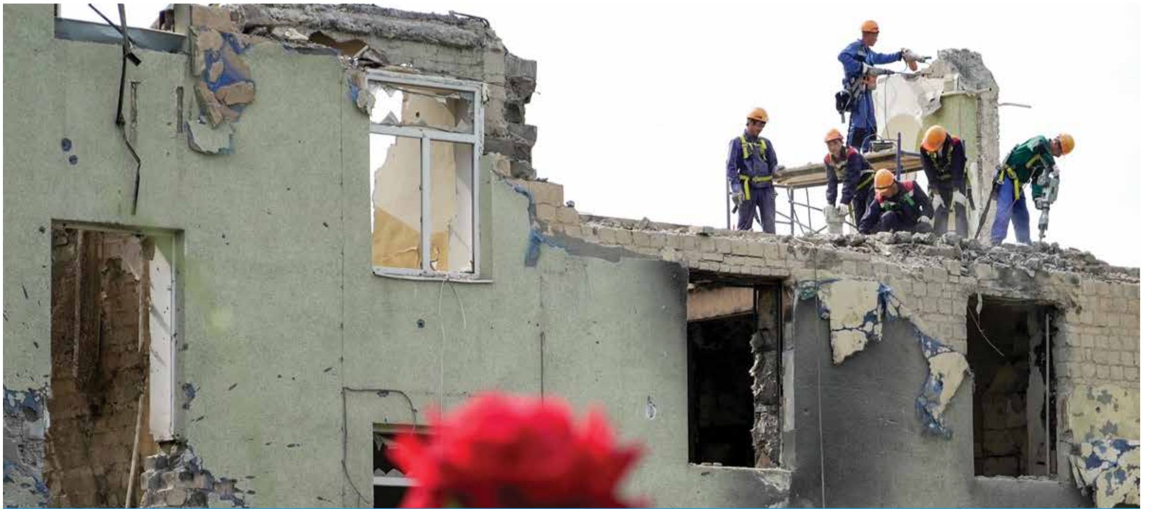
MARIUPOL: Workers fix partially destroyed building in the Russian-controlled Azov Sea port city of Mariupol in southeastern Ukraine. — AFP
