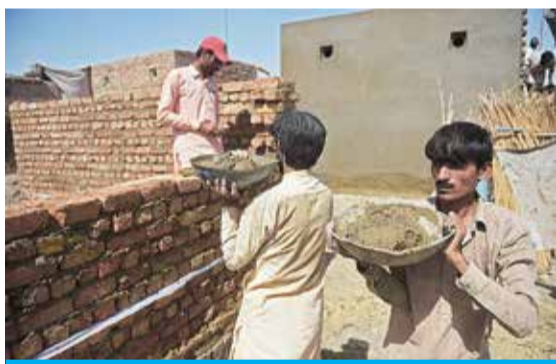
DADU: In this photograph taken on May 9, 2023, flood-affected victims rebuild their house in Dadu district of Pakistan. The government's pledge to rebuild the swathes of Pakistan ravaged by floods so they are resilient to future extreme weather has largely failed to materialize. — AFP
