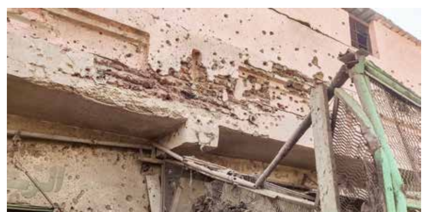
KHARTOUM: Bullet holes riddle the wall of a building at the Souk Sitta (Market Six) in the south of Khartoum on June 1, 2023. — AFP
