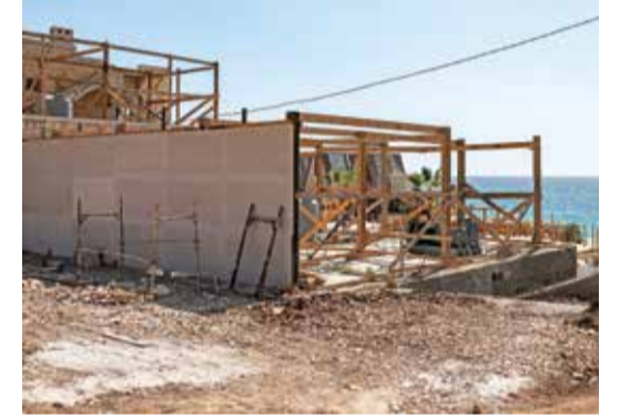
This picture shows a view of seaside facilities under construction in Lebanon's northern village of Thourm.
