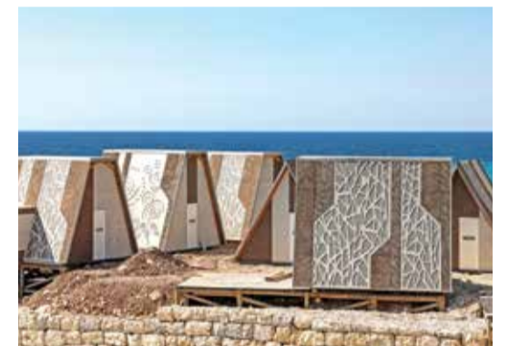
This picture shows a view of seaside facilities under construction in Lebanon's northern village of Thourm.
