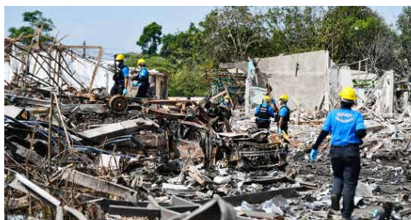
NARATHIWAT: Forensic personnel inspect the site of an explosion that ripped through a firework warehouse in Sungai Kolok district Narathiwat province on July 30, 2023. — AFP
