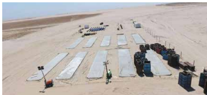
KUWAIT: These photos show construction work as part of the South Sabah Al-Ahmad project.
