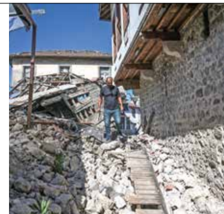
Gokhan Ergin, architect specialist on ancient buildings walks next to a damaged historical buildings as he inspects them, five months after a 7.8-magnitude jolt and its aftershocks wiped out swathes of Turkey's mountainous southeast at the ancient part of Antakya.
