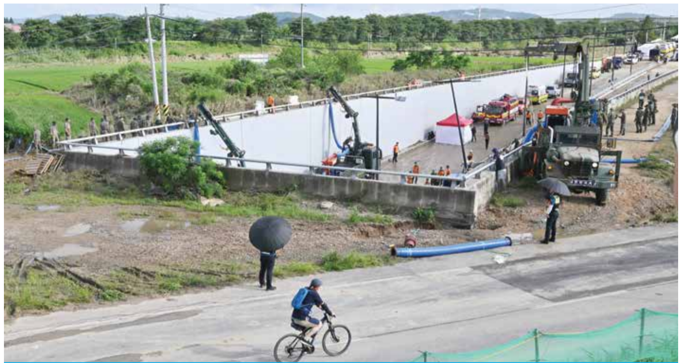
CHEONGJU: A man (bottom) rides a bicycle near an underground tunnel where 15 cars were trapped in flood waters after heavy rains in Cheongju. — AFP
