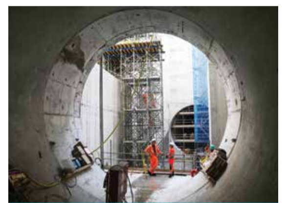
LONDON: Civil engineers work next to a 7 meter wide concrete tunnel at the Thames Tideway building site, in west London. London's existing sewerage network dates back to the second half of the 1800s. — AFP
