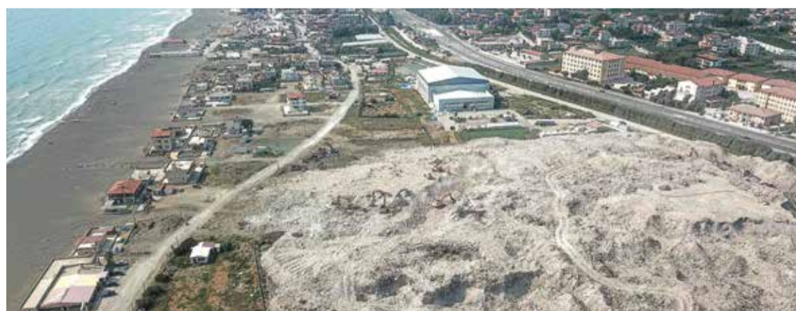
SAMANDAG: This aerial photograph shows excavators working on a landfill next to a beach in Samandag, in the south of the Hatay province. The excavator tore into the remnants of the damaged building in southeast Turkey, bringing them crashing down into a cloud of dust — the latest menace facing survivors of the deadly February quake that ravaged the region. — AFP
