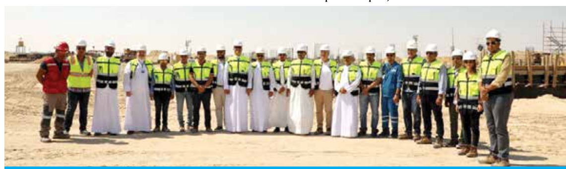
KUWAIT: Representatives from the GCC Interconnection Authority and the Kuwait Fund for Development inspect the construction site of the Wafra plant. — KUNA
