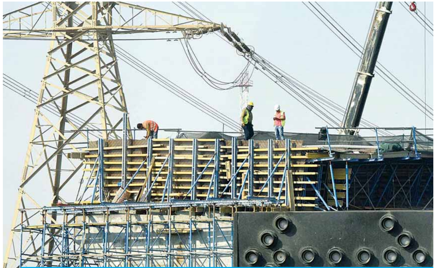
KUWAIT: Construction laborers work on a bridge project. —Photo by Fouad Al-Shaikh
