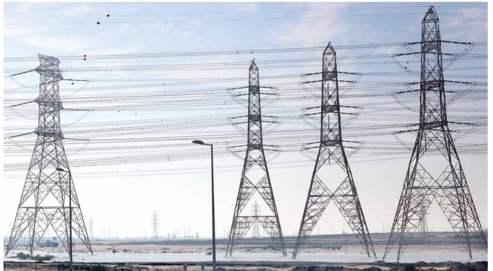
KUWAIT: Electricity pylons are seen against wisps of clouds. — Photo by Yasser Al-Zayyat
