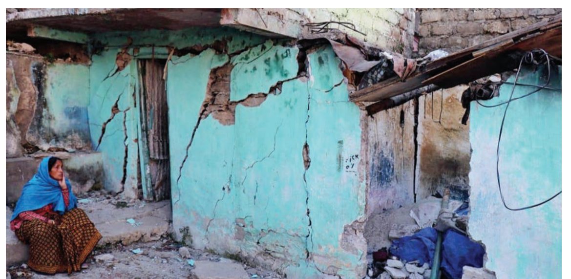
JOSHIMATH, India: A resident sits next to a cracked wall of her house in Chamoli district of Uttarakhand state on Jan 8, 2023. —AFP
