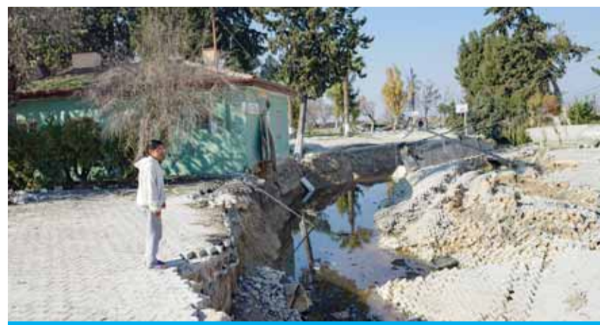
DEMIRKOPRU: A girl stands looking at the edge of a crack collapsed cobbled stoned street in Demirkopru, Hatay. —AFP photos
