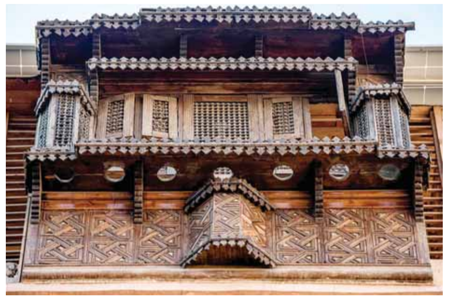
This picture shows a view of a mashrabiya, a balcony enclosed with carved wood latticework in traditional Islamic architecture, at the historical "Beit Yakan" house.
