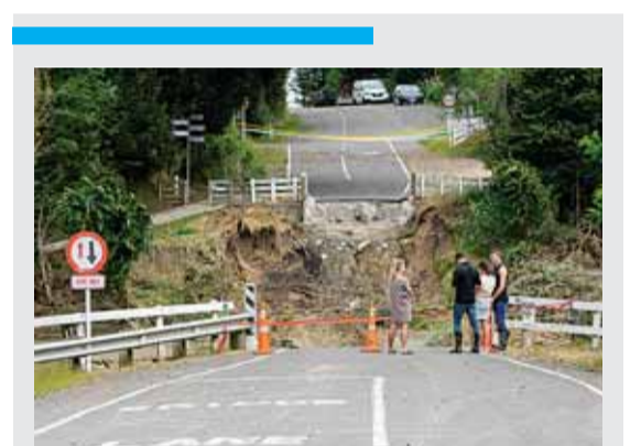
NAPIER: Photo shows the remains of the Puketapu Bridge that washed away during Cyclone Gabrielle near Napier on February 16, 2023. —AFP
