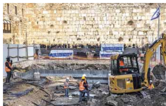
This file photo shows a view of construction works conducted by the Western Wall Heritage Foundation to build an underground floor at the Plaza of the Western Wall, the holiest site where Jews are allowed to pray, in the Old City of Jerusalem. — AFP photos
