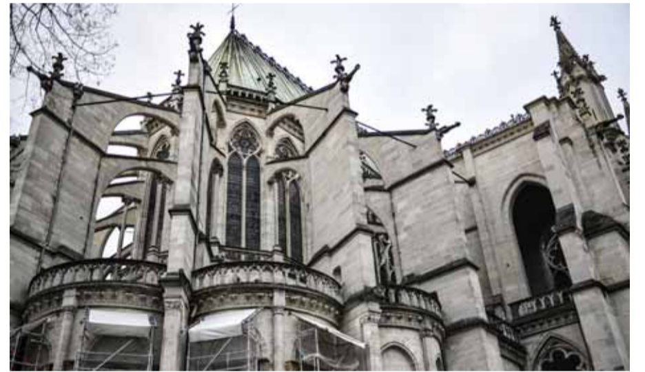
This picture shows the renovation site at the "Basilique de Saint-Denis" (Basilica Cathedral of Saint-Denis), in Paris' northern suburb of Saint-Denis.—AFP photos
