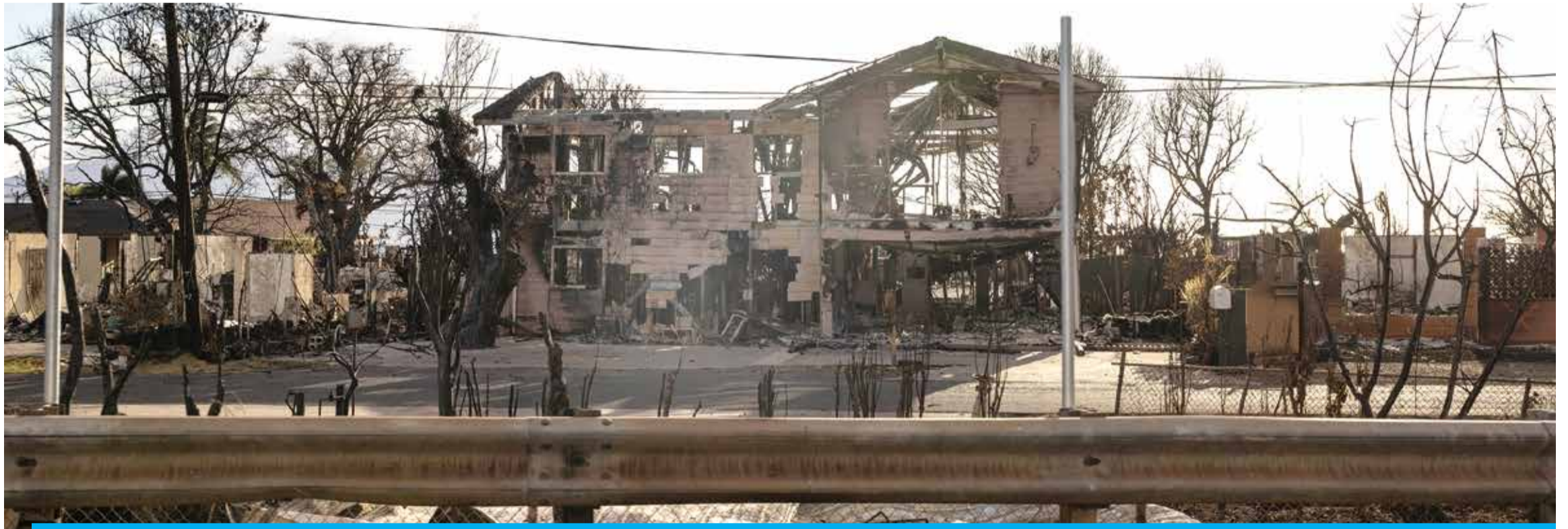
LAHAINA: The charred frame of a house is seen among the ashes of a burnt neighborhood in the aftermath of a wildfire, in Lahaina, western Maui, Hawaii on August 14, 2023. — AFP
