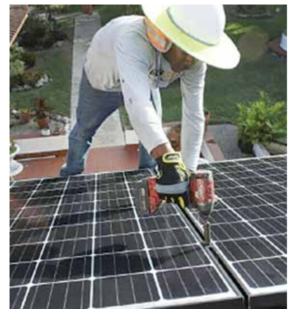
Solar panels are installed on the roof of a Florida house. — AFP
