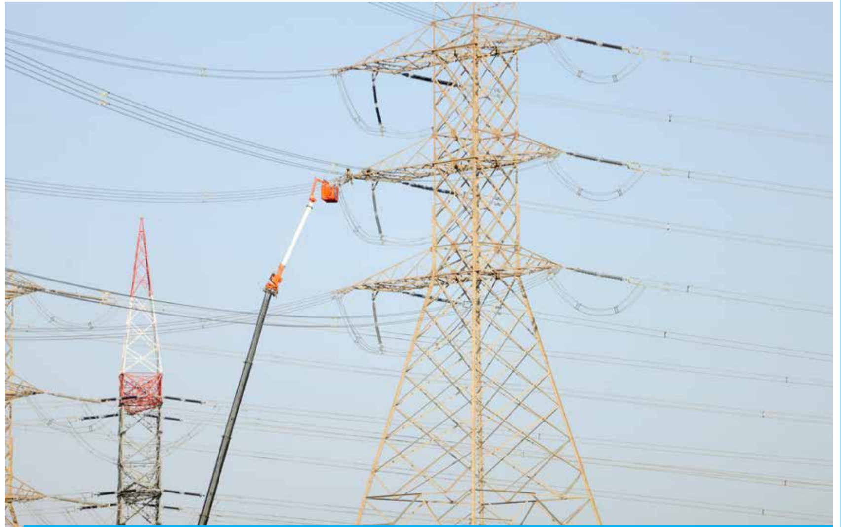
KUWAIT: Maintenance staff work on an electricity transmission tower off Fifth Ring Road. According to official sources, electricity consumption in Kuwait has eased marginally in the country this week after peaking it in July. On Friday, the maximum level of the temperature would be between 46 and 48 degrees Celsius during day time and 32 and 34 degrees at night, according to Kuwait Meteorological Department on Thursday. — Photo by Yasser Al-Zayyat
