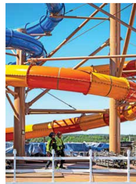
Workers walk at the construction site on a deck of the Royal Caribbean's new ship.
