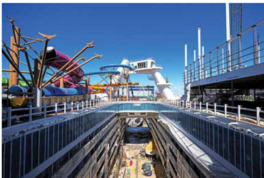
A general view shows the construction site of the Royal Caribbean's new ship 'Icon of the Seas' at the Turku shipyard in Finland's southwest coast.
