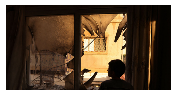
NABLUS: A youth inspects the remains of a house demolished by Zionist soldiers at the Asker camp for Palestinian refugees in the occupied West Bank on Aug 8, 2023. — AFP
