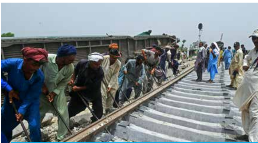
NAWABSHAH, Pakistan: Railway workers repair a damaged track, a day after the derailment of a passenger train in Nawabshah on August 7, 2023. — AFP
