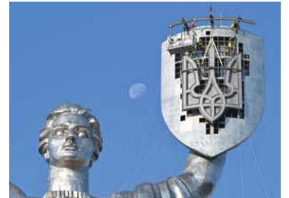
KYIV: Steeplejacks operate to install the Ukrainian official coat of arms, also known as the tryzub, replacing the coat of arms of the former Soviet Union which was previously removed, on the shield of the 62-meter (102 meters with pedestal) Motherland Monument in Kyiv, on August 6, 2023. — AFP
