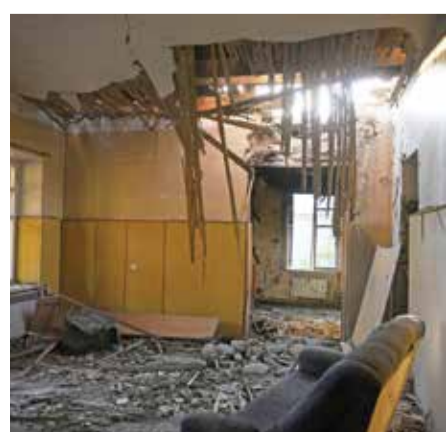
A view of a guest house destroyed in artillery fire from Azerbaijan in the town of Jermuk on September 15, 2022.
