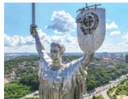
This aerial view shows the Motherland Monument as steeplejacks dismantle the coat of arms of the former Soviet Union from the shield of a 62-meter (102 meters with pedestal) Motherland Monument in Kyiv.
