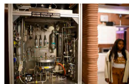
The oxygen generator system inside of CHAPEA's Mars Dune Alpha.
