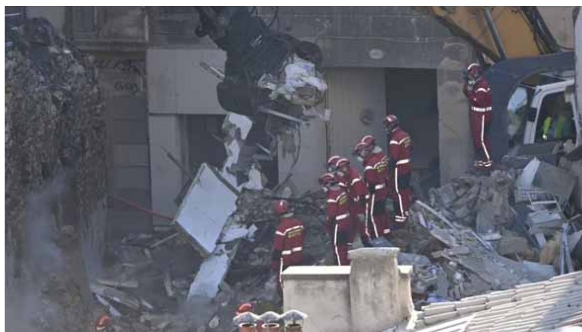
MARSEILLE: Firefighters stand aside as an excavator clears rubble at 'rue Tivoli' after a building collapsed in the street, in Marseille, southern France. — AFP
