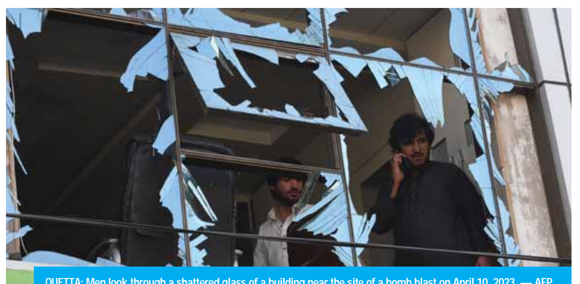
QUETTA: Men look through a shattered glass of a building near the site of a bomb blast on April 10, 2023. — AFP
