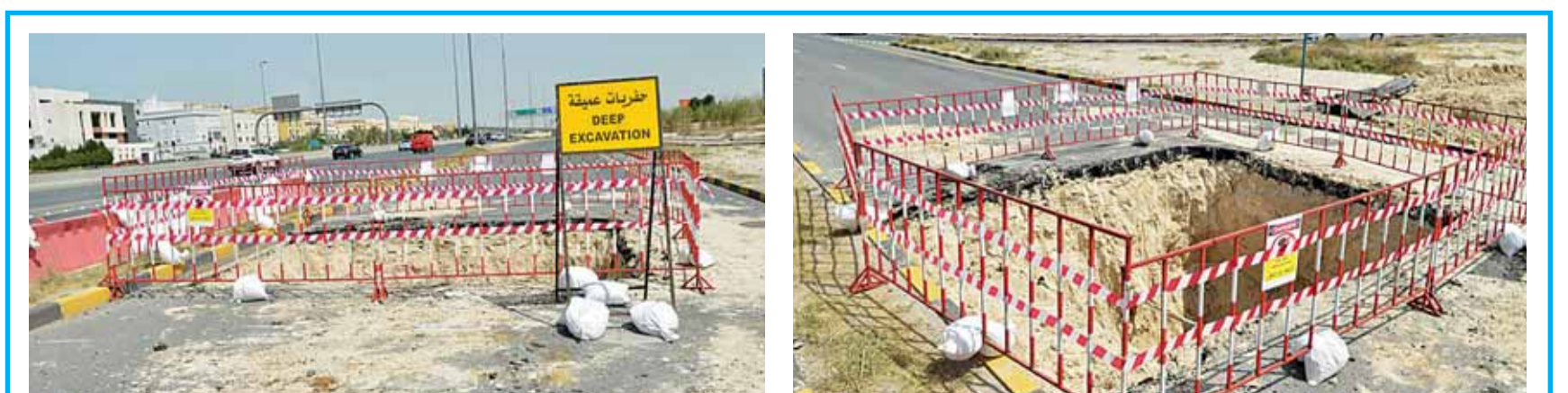
KUWAIT: The Public Works Ministry is examining the reason behind the sinkhole on the Fourth Ring road near Andalus area. The emergency teams rushed to the site and cordoned off the area to prevent any accident. —Agencies
