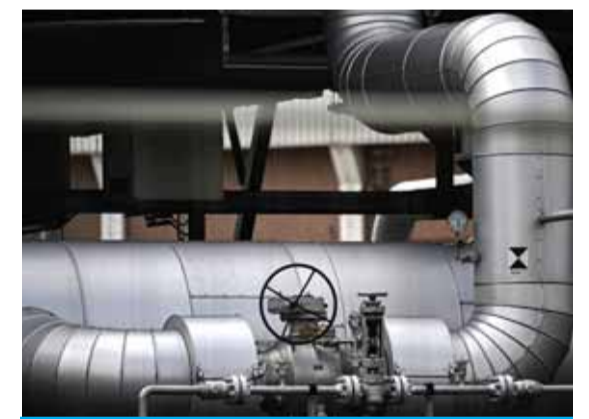
WERNE, Germany: This file photo shows pipes and pressure gauges for gas at the Open Grid Europe (OGE), one of Europe's largest gas transmission system operators, in Werne, western Germany. — AFP
