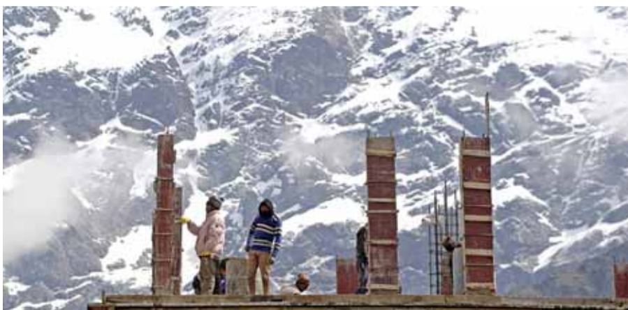
Indian laborers work on a construction site with a view of the Himalayas in an area that was hit during the deadly floods in Rudraprayag District in northern Uttarakhand state.— AFP
