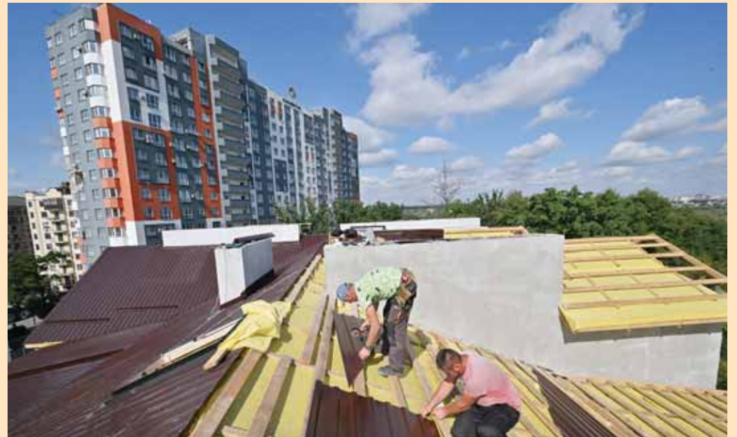
IRPIN, Ukraine: Workers repair the roof of an apartment block partially destroyed by shelling in the town of Irpin, Kyiv region. Over a hundred residential blocks in Irpin - dubbed a "hero city" by President Volodymyr Zelensky for holding Russian invaders on their way to the capital - were badly damaged by shelling. —AFP
