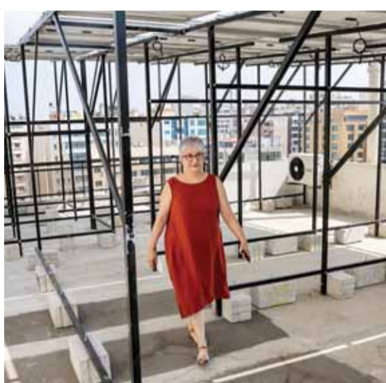
BEIRUT: Lebanese homemaker Zeina Sayegh walks beneath the solar panels she installed atop her apartment building in Lebanon's capital Beirut.
