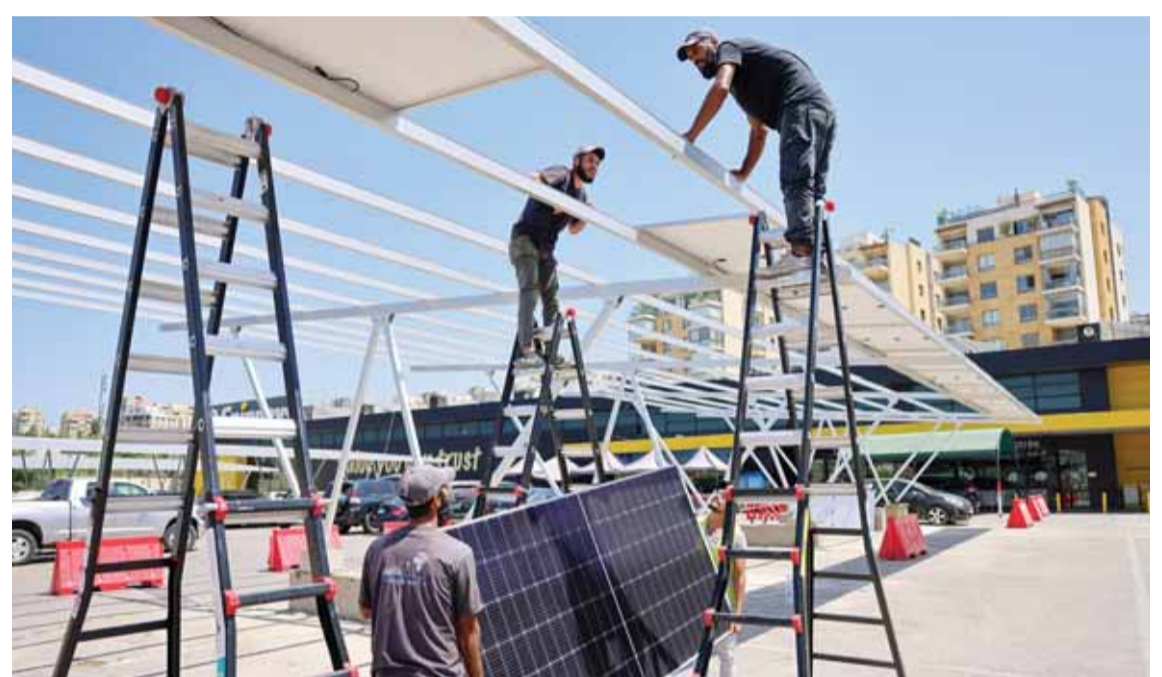
BYBLOS, Lebanon: Workers install new solar panels as shades above vehicles in the parking garage of a shopping mall in the city of Byblos in northern Lebanon on August 26, 2022. — AFP photos
