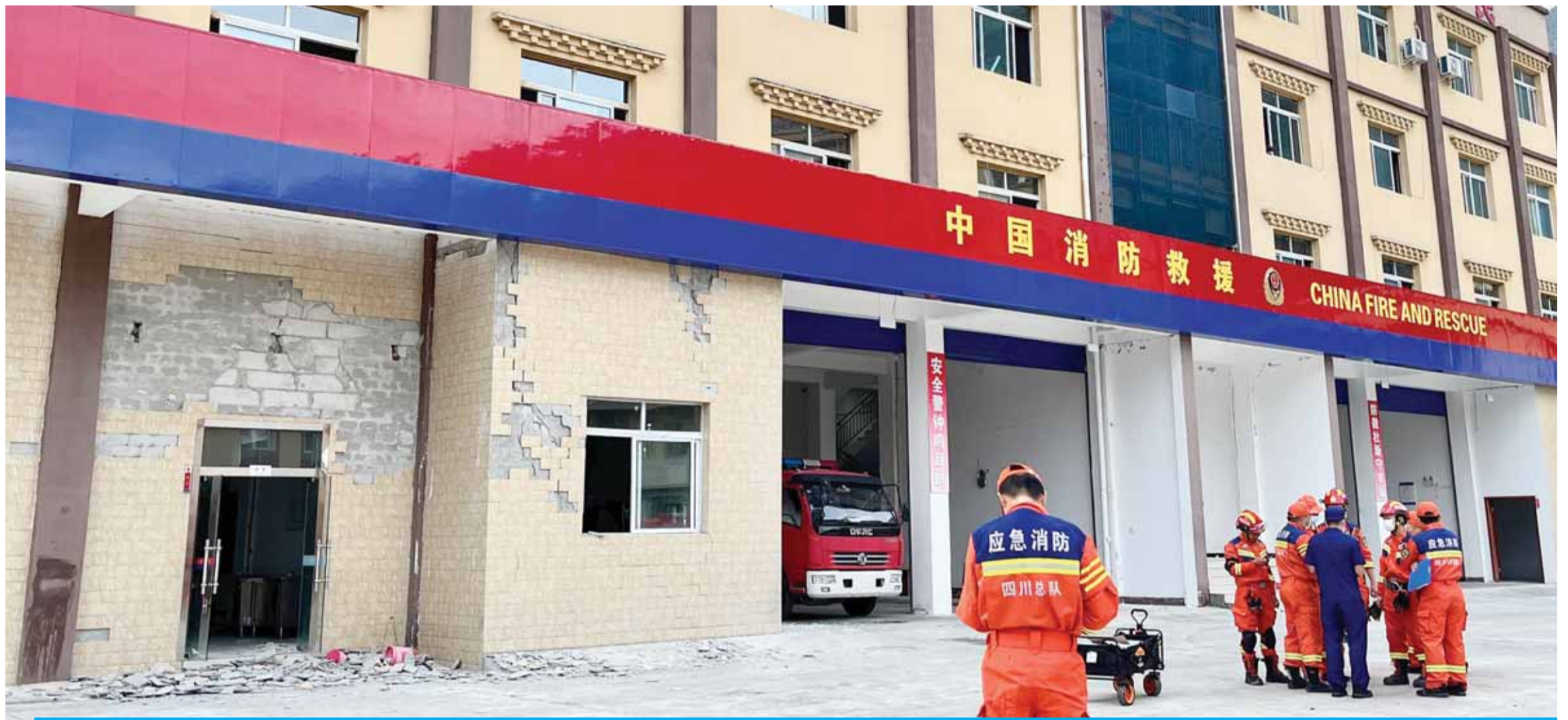
HAILUOGOU, China: Firefighters gather near a damaged wall of a fire station after a 6.6-magnitude earthquake in Hailuoguo in China's southwestern Sichuan province on September 5, 2022. —AFP
