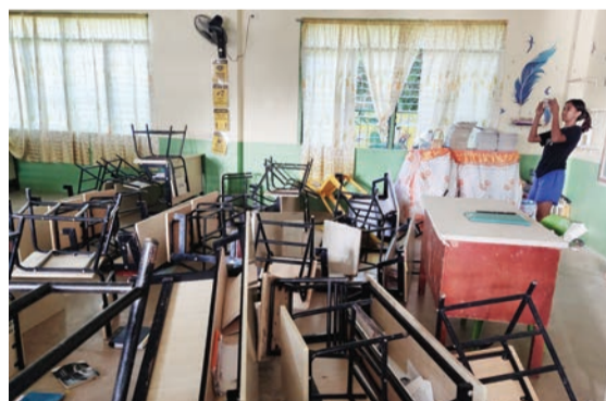
LAGAYAN: This handout photo taken and released by Ralf Jo Largo on October 26, 2022 shows a damaged classroom of Pulot National High School in Lagayan, Abra province, after a 6.4-magnitude earthquake hit the northern Philippines. — AFP
