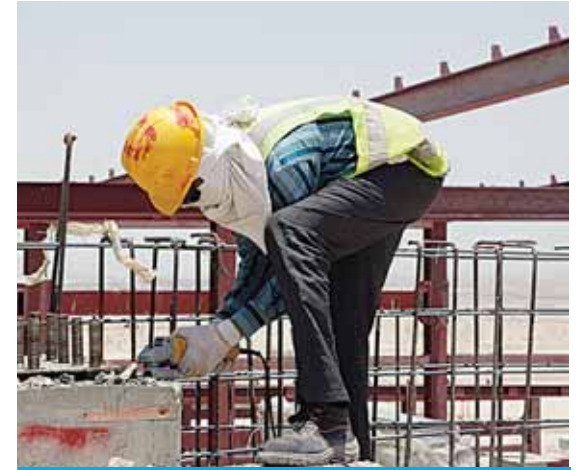
KUWAIT: A construction worker is seen at a site in this illustrative file photo.
